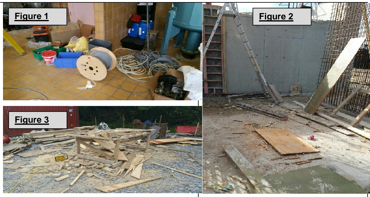
Figures 1-3 above were taken during IW HSQE Inspections on Irish Water sites and demonstrate examples of poor housekeeping practices.
