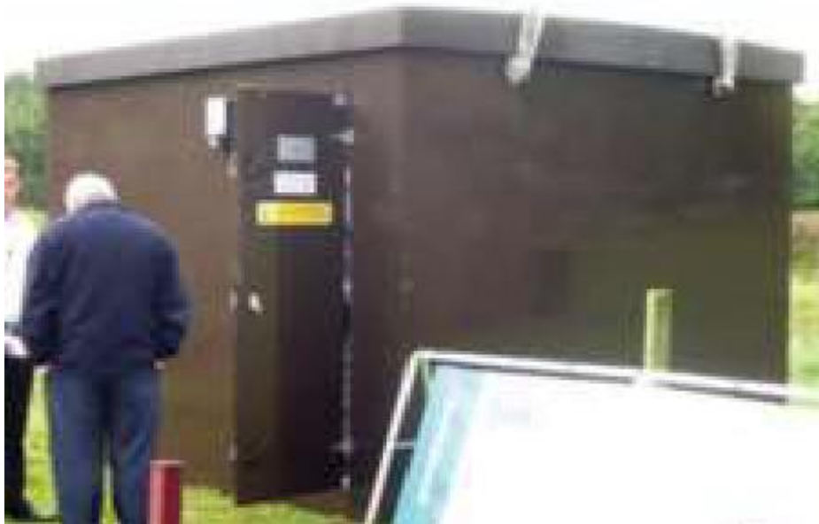
Figure 3 Typical orthophosphate dosing unit
