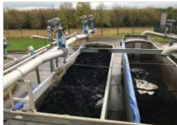
Figure 3.20: Bunlicky WwTP Dewatered Sludge Storage
