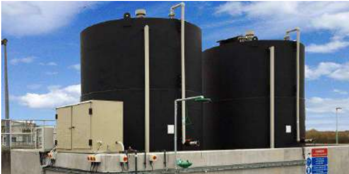
Figure 3.17: 2 no. 20m 3 tanks installed at Bunlicky WwTP (courtesy – Silotank)
