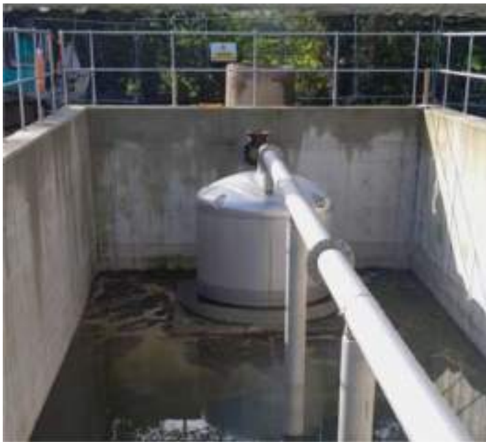
Figure 3.2: Lifford WwTP CWF Storm Flush Image 1
